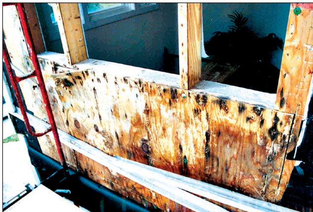
Figure 3 – Deterioration of sheathing and framing from water leakage at window openings.
