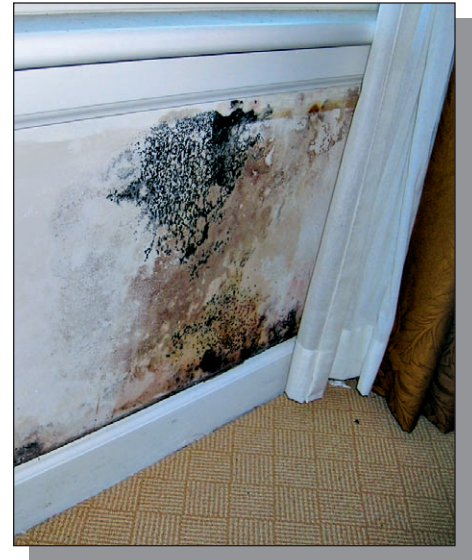
Figure 4 – Mold growth on gypsum wall
