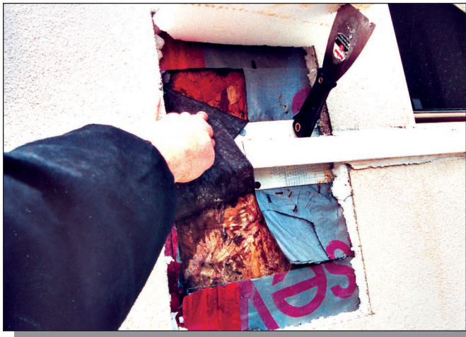
Figure 2 – Example of water damage due to water penetration through a polymeric WRB membrane.
