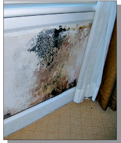
Figure 4 – Mold growth on gypsum wall
