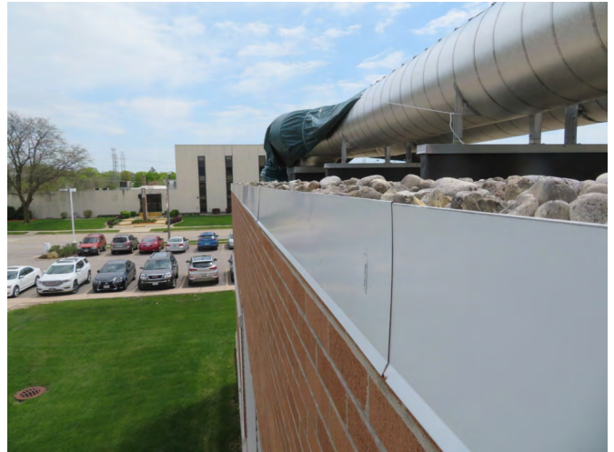
Photo 1: Edge metal must be higher than ballast (2-inch minimum). (Raths Raths & Johnson photo)
